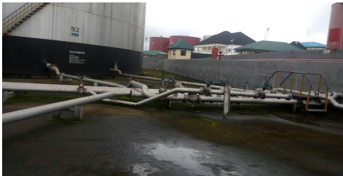
PLATE 2: The pipes of the inlet lines where products are discharged from the vessels to the tank.
