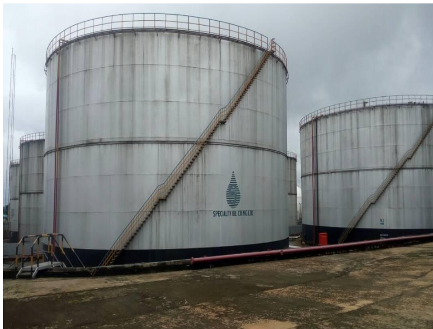
PLATE 1: Tank farms at Calabar jetty
